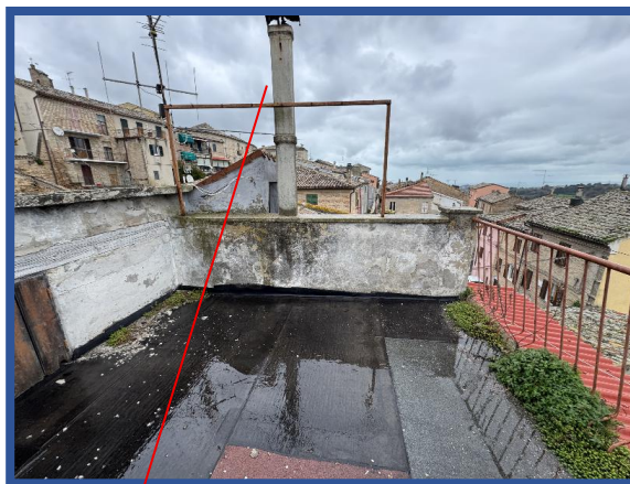
CANNA FUMARIA IN AMIANTO
