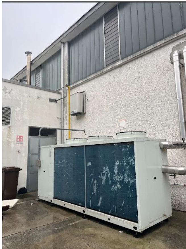
D.38. CHILLER EMICON
